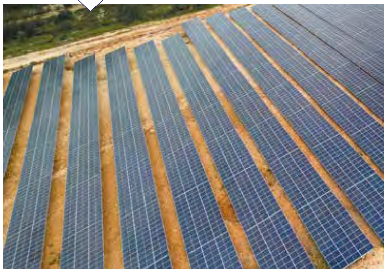
Caveirac photovoltaic solar park
